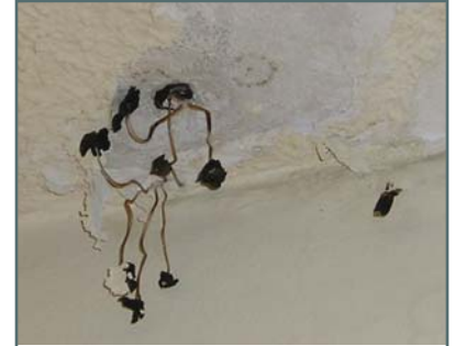
Mold Remediation Needed – Hazardous to your health mushrooms growing out of a ceiling due to water intrusion - Photo by Travis I. Irving Staff Scientist at H2M
